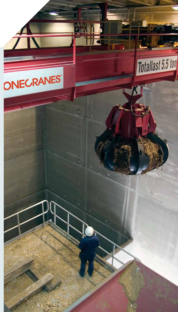
London, UK, 2 units 25-ton capacity Goliath cranes to lift waste containers from barges to trucks.
